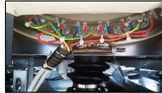
Electric heating elements in front
